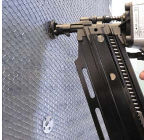
Lath and plaster washers attaching lath over continuous insulation using a Bullseye magnetic adaptor on a nail gun.
