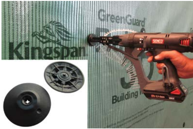
Rapid attachment of building wrap to steel studs using auto-feed screw guns with custom Grip-Lok nose cup adaptor with 2 inch diameter air sealing washers.
