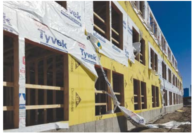
This is what can happen when insufficient fasteners or installation techniques are used to attach building wrap. Thousands of dollars in repair work on this project could have been avoided if proper fasteners and large diameter plastic washers had been utilized during the installation.
