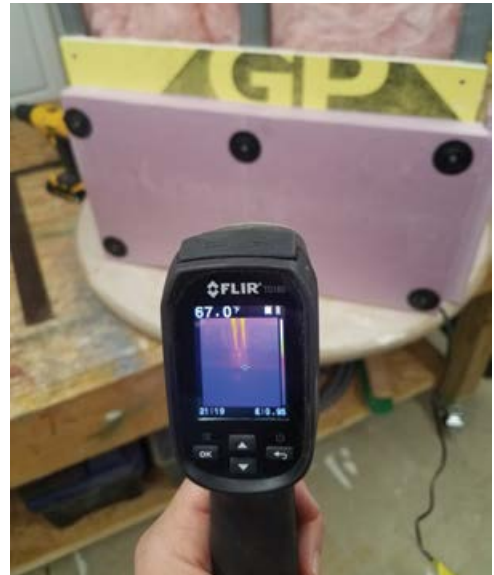
A small heater is placed inside the mini "hot box" structure. FLIR infrared thermal-imaging camera clearly shows the temperature gradient and thermal-bridging of the steel studs, compared to the lower section of the wall covered with continuous insulation.
